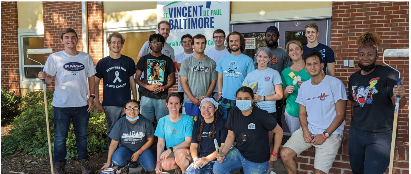
A team of 20 Whiting-Turner interns prepare a basement for a fresh coat of paint at Hannah More.
